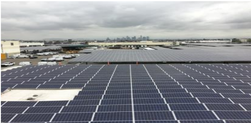
US Postal Service Solar, 10 MW
