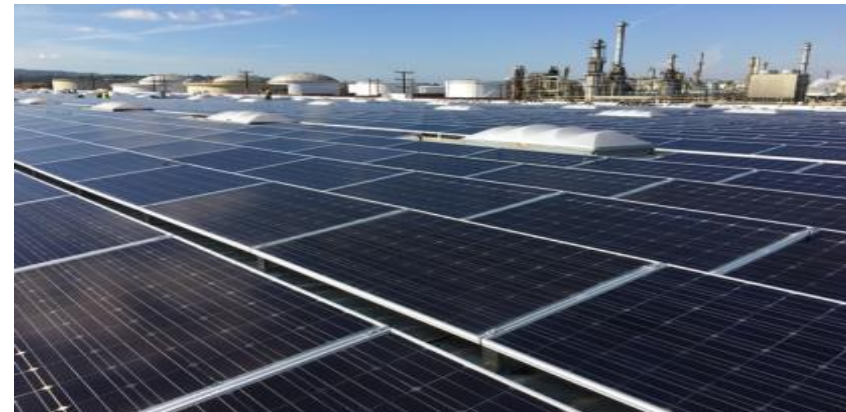
Westmont Solar, 15 MW
