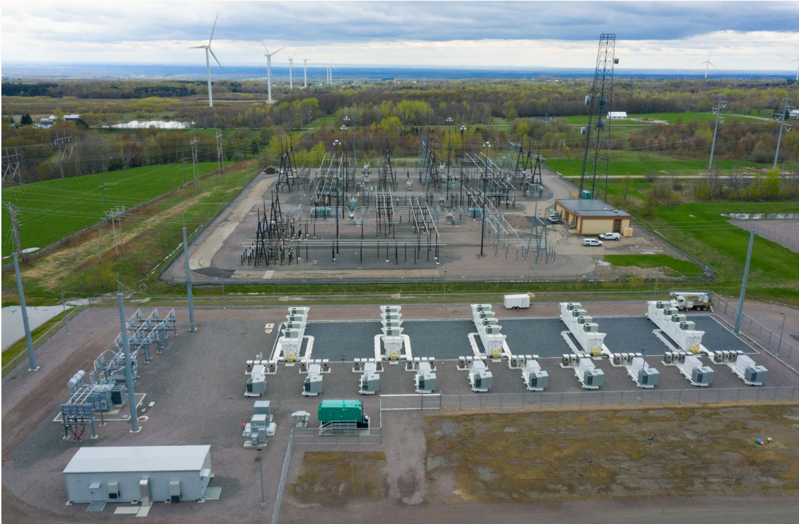
Drone view of the Northern New York battery storage project, with the Willis substation adjacent to the facility
