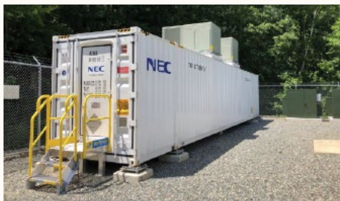
The installed NEC Battery Storage Container and Step-Up Transformers
