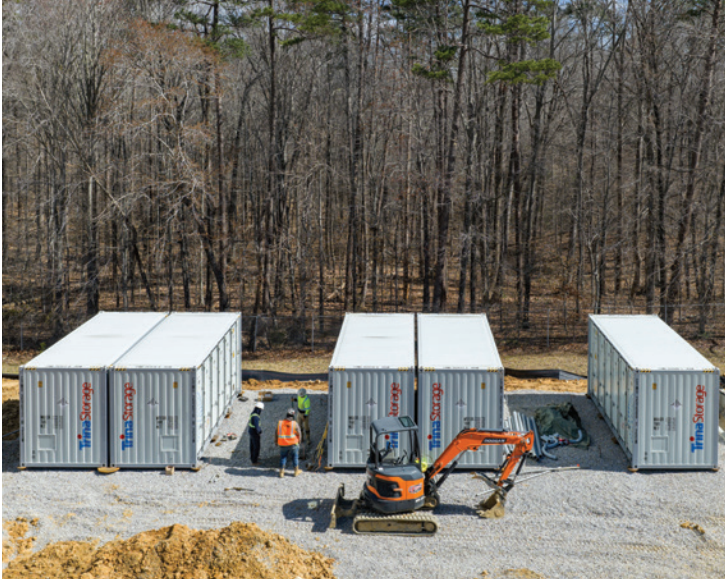
Photo courtesy Sanjay Suchak/Lightshift Energy
