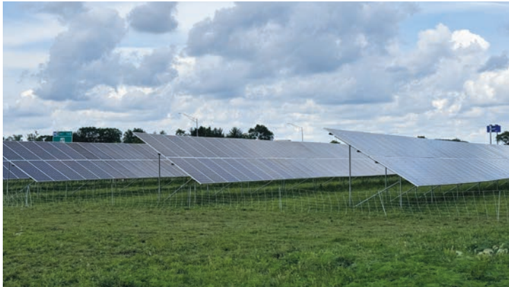
The SunSmart Ames community solar project.
